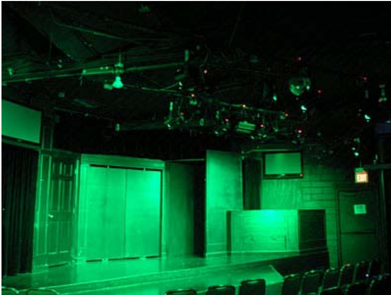
Brave New Workshop has converted its stage lights to LEDs, which has helped to cut its electric bill by 73%.
